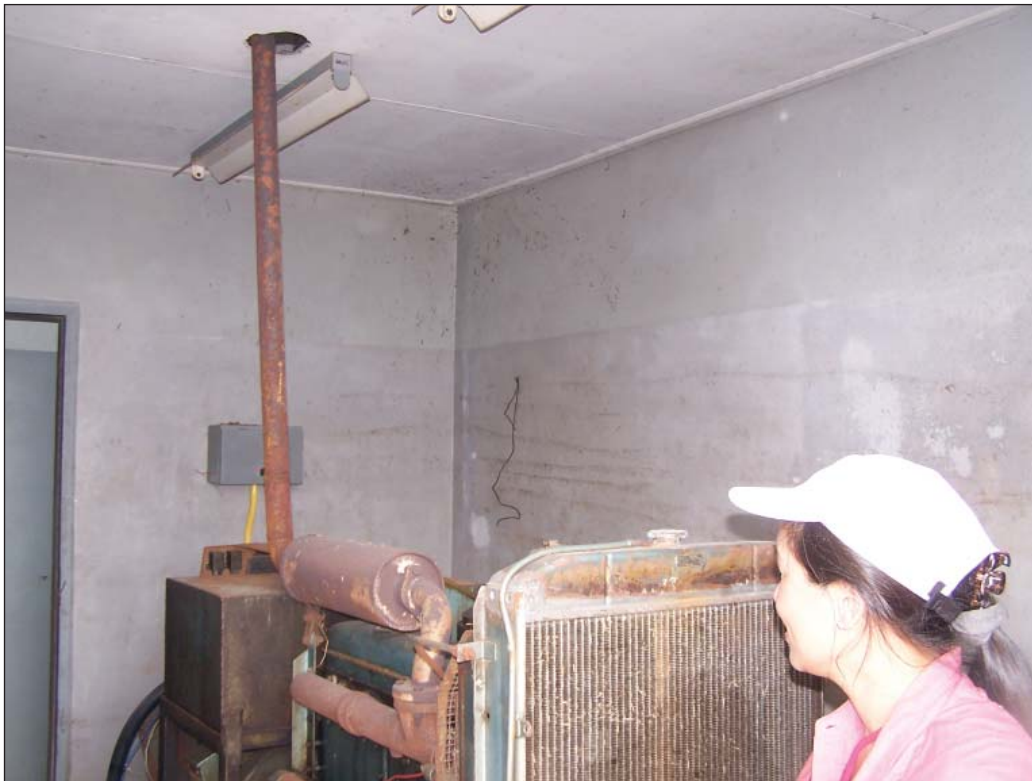
Fig. 10.1 Emergency generator at the water treatment plant. Note the high water marks on the walls and the debris in the radiator grill.
