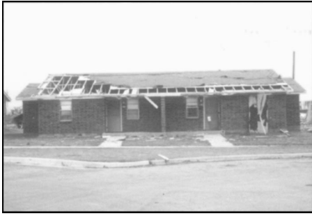
Fig. 1. Building envelope damage may result in total insured loss
