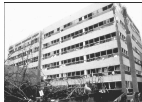
Fig. 4. Roof gravel broke fully tempered glass on building in Cutler Ridge, Fla.
